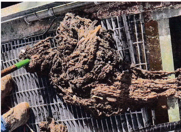
Image of old wipes and grease stuck in the sewer system.
